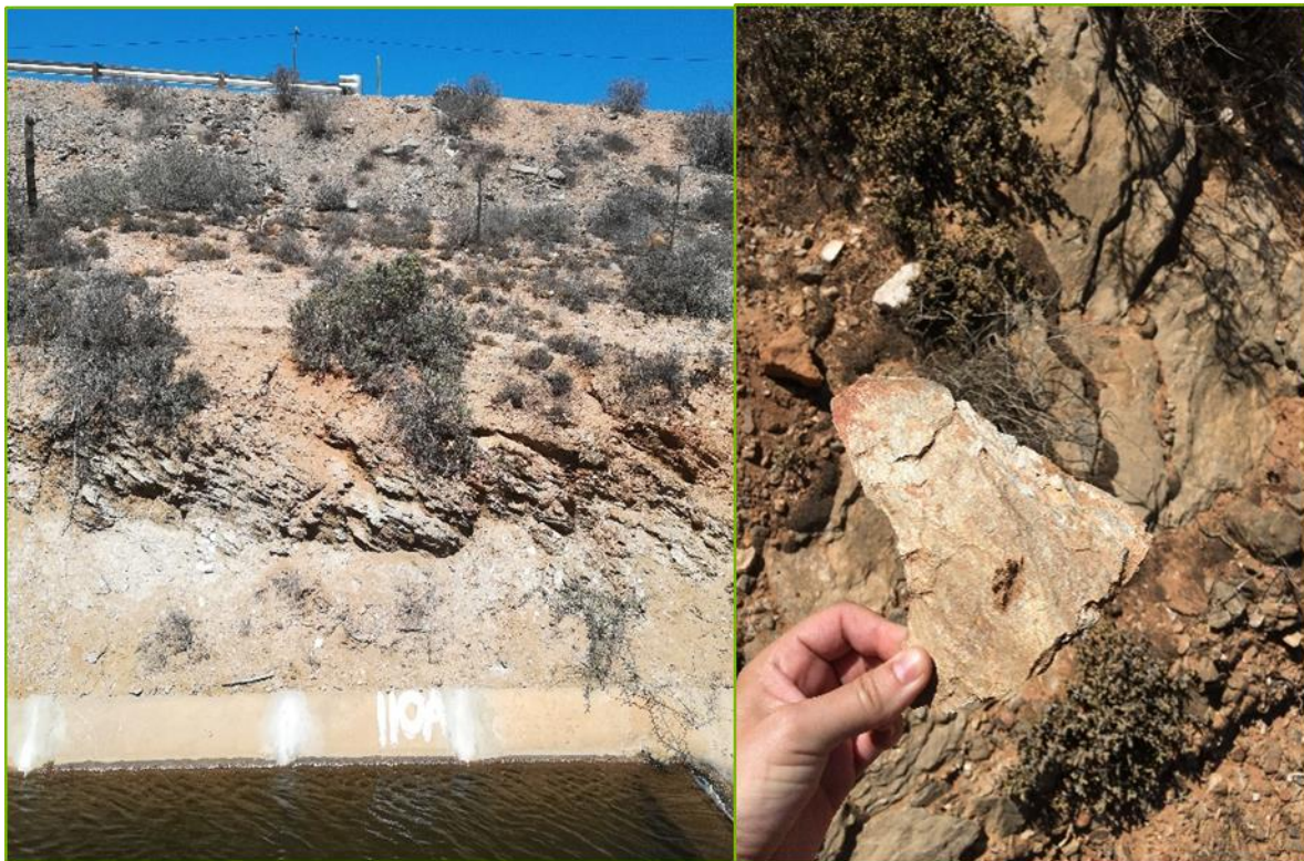
Figure 16: Exposed schist dipping between 30° and 40° as encountered along the existing left bank canal
